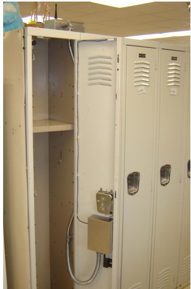
Fig. 8.23. Locker Unit and Power Supply.
